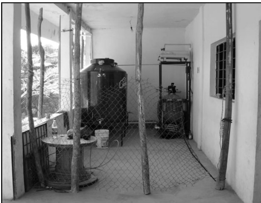
Figure 2 UVWaterworks installation in Cuilutla, Mexico. Unpurified river water from the community piped-water system enters the UVW system from storage tanks located on the roof. This water then passes through the filtration system (tanks located bottom right) and then through the UV purification system (box located top right). Clean water is then stored and dispensed to community members through a recontamination resistant tank and faucet system (tank left)
